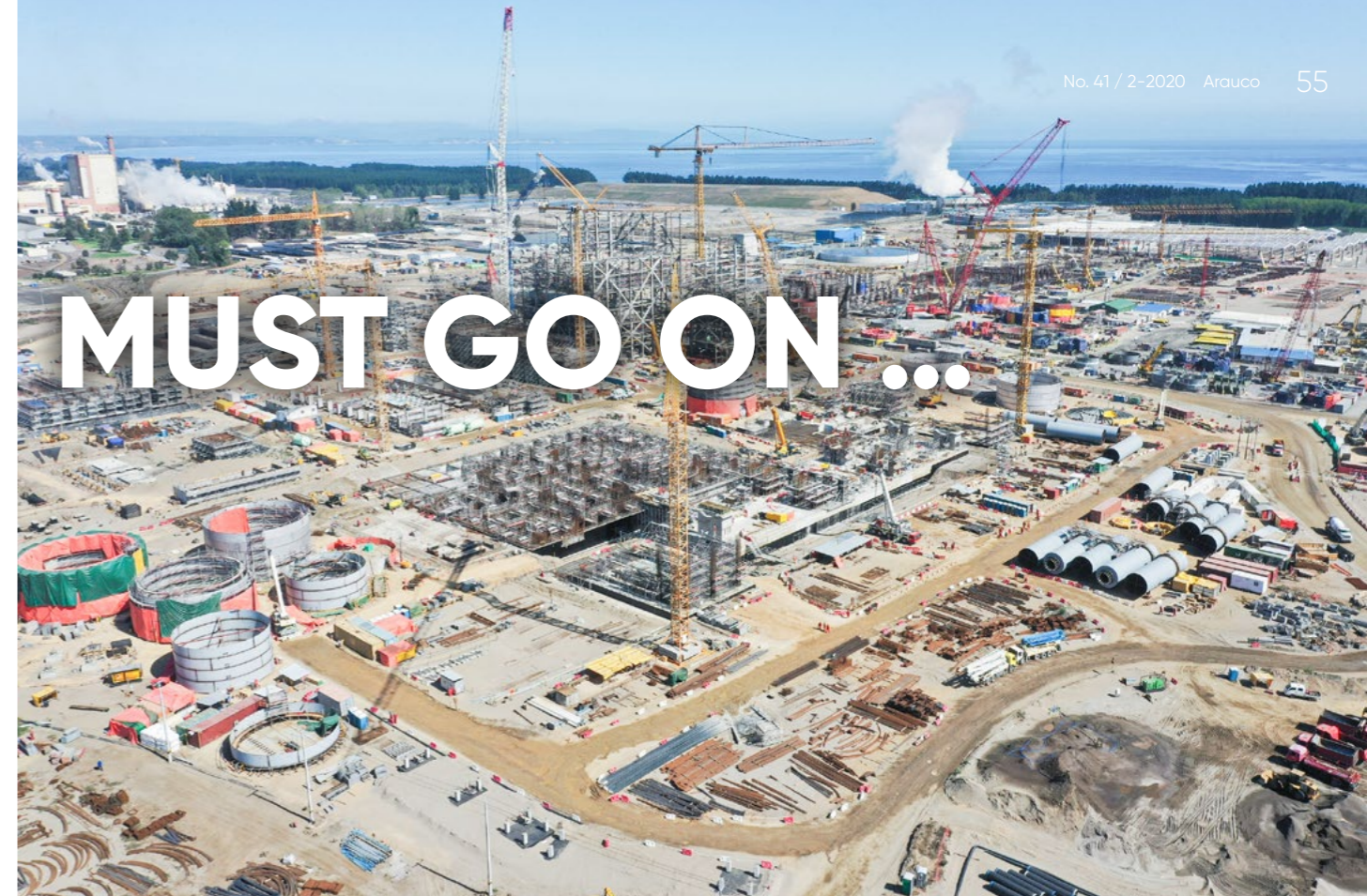
Work continues on civil works at the MAPA project in Chile; the mechanical installation stage is next.
